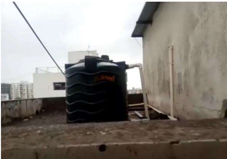
Water storage tank on roof
