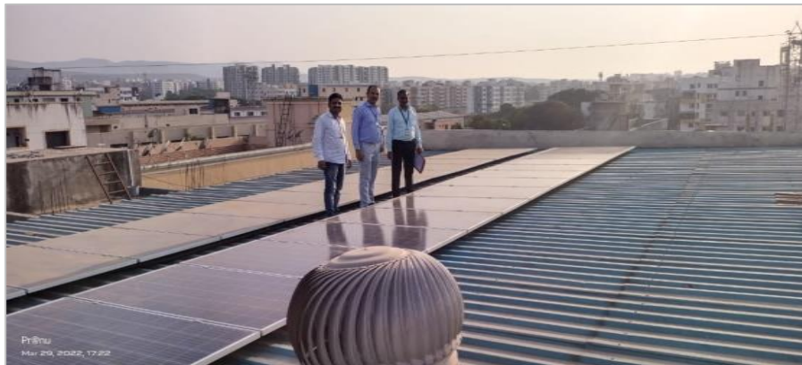
Energy efficient fan and solar roof top
