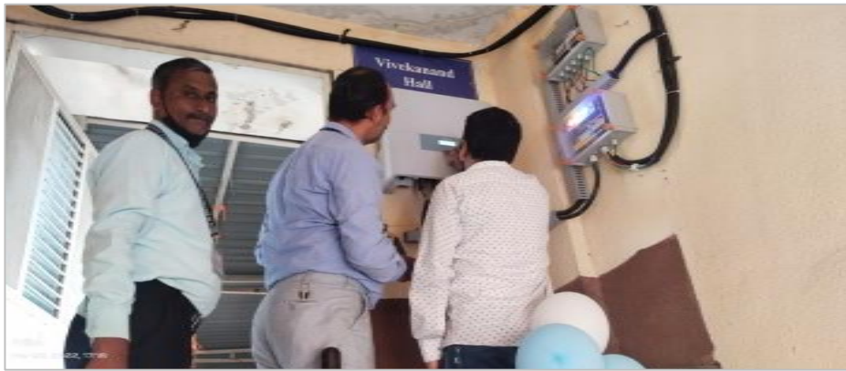
Net metering device in the premises
