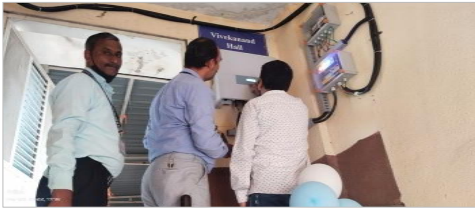
Net metering device in the premises
